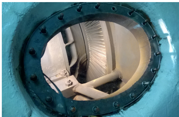
Figure 8.14: Inspection window of one of the low-pressure turbines (power approximately 25 MW) of the aircraft carrier USS Hornet launched in 1943.
